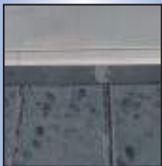
Before - Open seams and deteriorated surface on modified bitumen membrane on sloped wall
