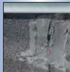
Before - Open joint in modified bitumen flashing on built-up roof system
