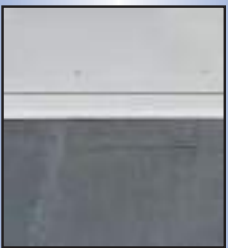
After - Reinforced open seams by using a three-course flashing repair system including a fibrated asphalt emulsion coating.
