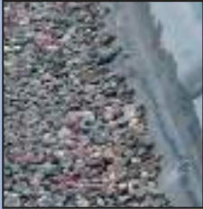
Before – Tenting of EPDM membrane at perimeter wall due to loss of attachment of membrane to base tie-in.
