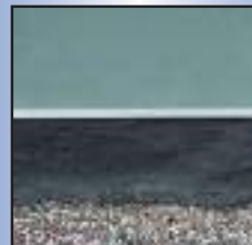
After - Repaired open joint in flashing by using the three-course flashing repair method.
